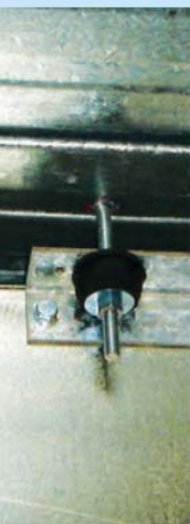
Figure 14(a). JetVent installation using anti-vibration mounts
