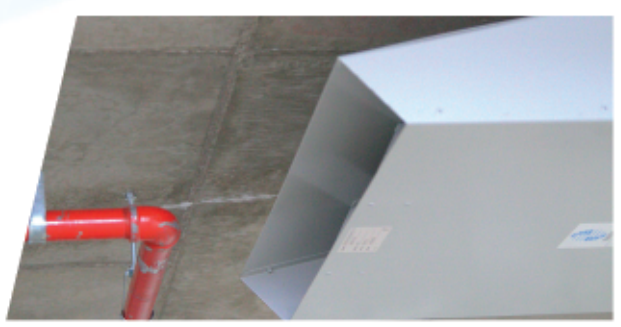
Figure 10(d). Pipe work can impede fan throw
