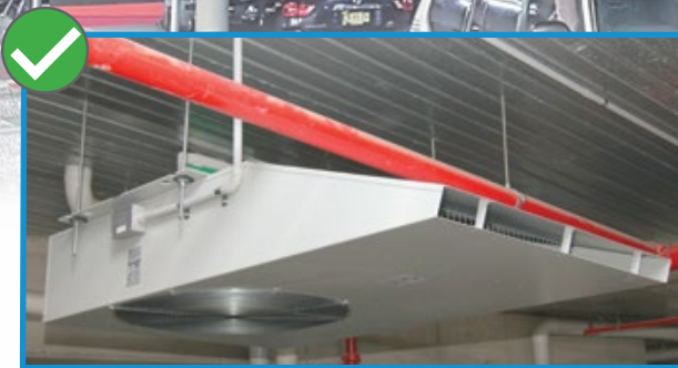
An example of how to avoid clashes with pipework
